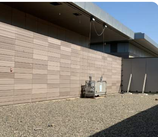
Fig. 1 - Exterior Wall Condition of Mechanical Room
